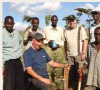
John Alexander completes the final standpipe, watched by Roger and the rest of the squad
